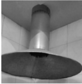
Figura VIII.18 Campana extractora del local.
